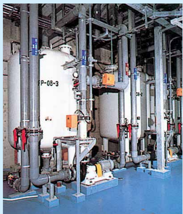
▲Eslon Valves for Aquarium piping.
